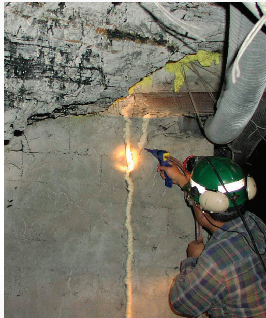
REPAIR DAMAGED BLOCK STOPPINGS
